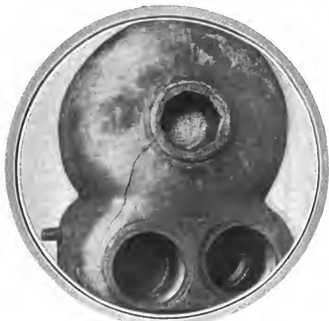
Fig. 3—Showing a cracked water jacket which will allow the cooling water to run away
